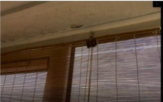
Photo 3.31: Peeling of paint underside of roof slab in living room of flat [redacted]
