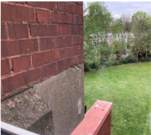
Photo 3.12: Crack in top corner of beam facing green adjacent stairwell to flats 247-248. Visible from landing window.
