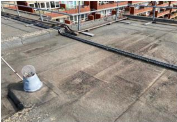
Photo 3.1: Roof surface showing evidence of rainwater ponding
