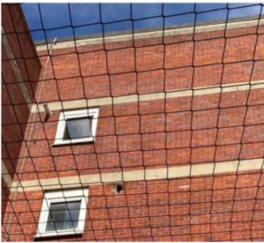
Photo 3.10: Side elevation facing Ball Court showing hole in brickwork underside of 4 th floor slab.
