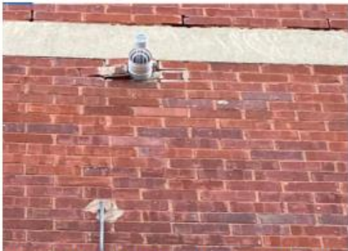
Photo 3.36: Dislodged bricks around boiler exhaust on Shuttleworth Road elevation to flats 63-65
