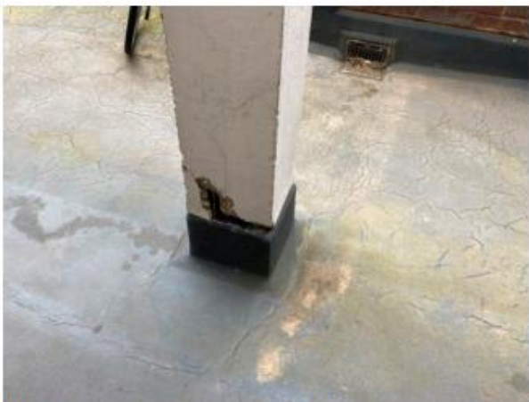
Photo 3.17: Crack and spalling of concrete at base of column in front of sub entry to flats 249-251 on 4 th floor walkway.
