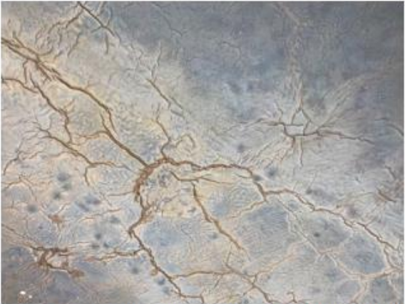
Photo 3.25: Severely cracked asphalt on 4 th floor walkway
