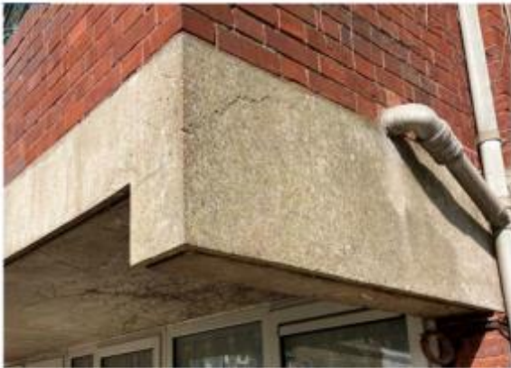
Photo 3.33: crack in repair work to concrete beam in the past
