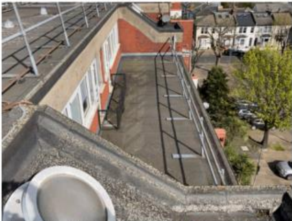
Photo 3.3: 5 th floor Communal Balcony Evidence of rainwater ponding
