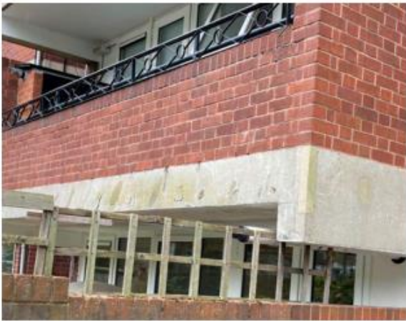
Photo 3.27: Multiple cracks on face of concrete slab at 1 st floor, LHS of Entrance C on Bullen Street
