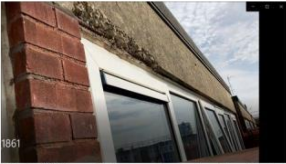
Photo 3.32: spalled concrete underside of balcony lintol in flat [redacted]
