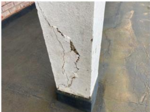
Photo 3.19: Column fractured at bottom on 4 th floor walkway, adjacent entry to flats 165-170
