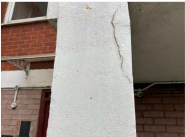
Photo 3.16: Crack at the top of column in front of sub entry to flats 249-251 on 4 th floor walkway
