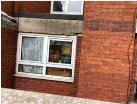
Photo 3.38: Concrete spalling at bottom RHS corner of lintel over storage window
