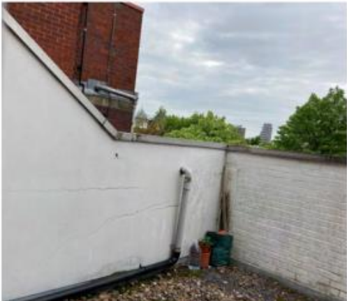
Photo 3.4: 4 th Floor Communal Terrace opposite flat 202 showing cracking of side wall
