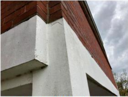
Photo 3.39: Crack at top corner of column on 4 th floor walkway adjacent to entrance to flats 264-269
