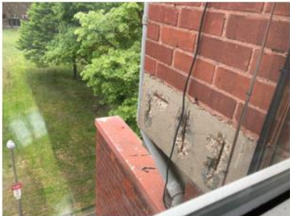
Photo 3.14: Spalling of concrete on beam surface exposing reinforcement, facing green adjacent stairwell to flats 216 and 217. Visible from landing window.
