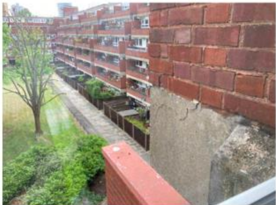
Photo 3.13: Crack in top corner of beam facing green adjacent stairwell to flats 208-209. Visible from landing window.
