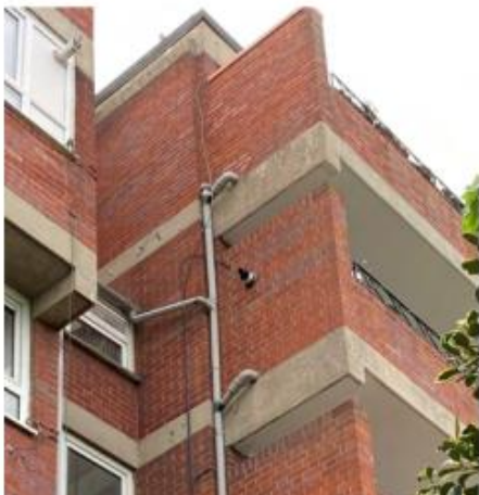
Photo 3.28: Cracks in recessed bay on 4 th and 5 th floor slab/beam faces adjacent downpipe between Flat 77 and Entrance B on Bullen Street
