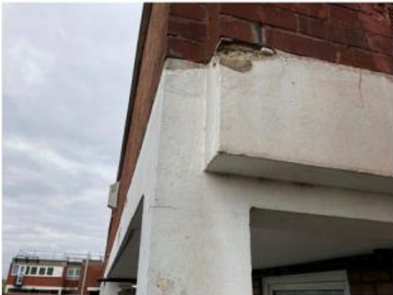
Photo 3.22: Spalling of concrete at top corner of beam. Same beam in photo 21
