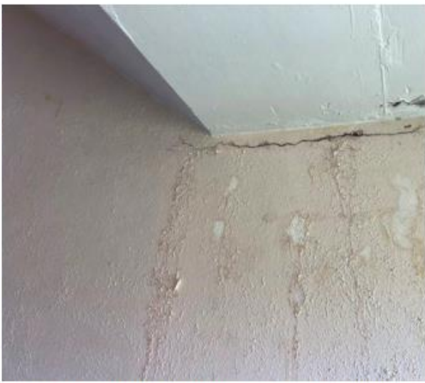
Photo 3.8: Sloped Roof over stairs to sub entry to flats 247-248: Horizontal crack in wall beneath slab. Evidence of moisture ingress.
