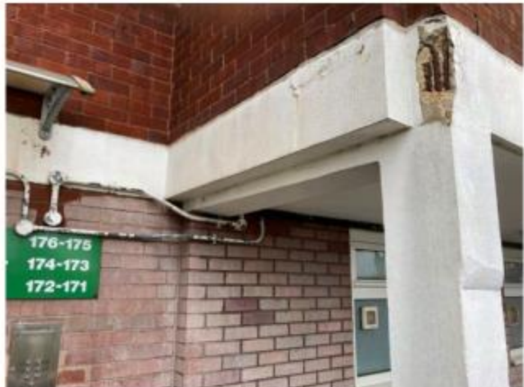
Photo 3.20: Severely spalled concrete exposing reinforcement at beam and column joint on 4 th floor walkway adjacent entry to flats 171-176
