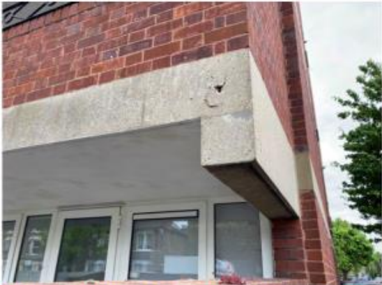
Photo 3.29: Cracked and spalled concrete on face of 1 st floor slab at corner of Bullen Street and Shuttleworth Road junction.
