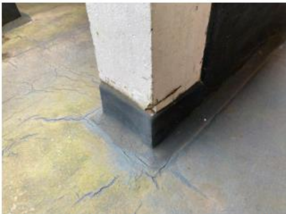
Photo 3.15: Crack in base of column on 4 th floor walkway in front of sub entry to flats 252-257
