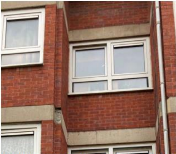
Photo 3.9: 2 nd floor slab adjacent flats 128 and 129 Loss of concrete at slab recess leaving brickwork unsupported.
