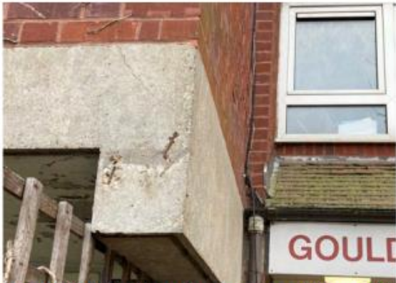
Photo 3.37: Spalling of concrete and diagonal top crack in beam LHS of Entrance B on Bullen Street
