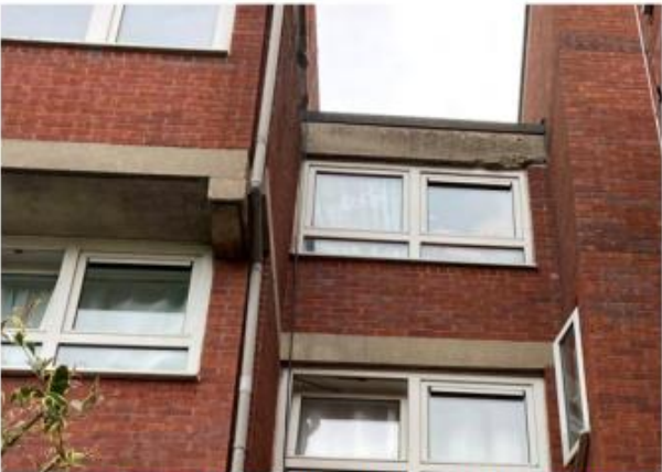
Photo 3.26: Spalled concrete in bottom corner of top lintol in recessed bay facing inner green above flat 127
