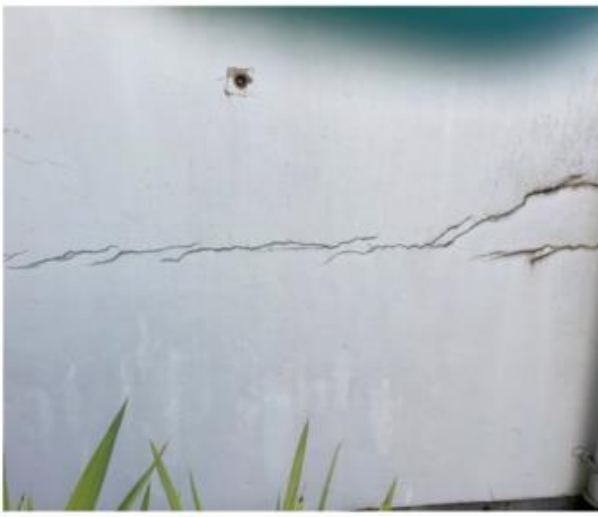
Photo 3.6: 4 th Floor Communal Terrace opposite flat 232 showing crack in side wall
