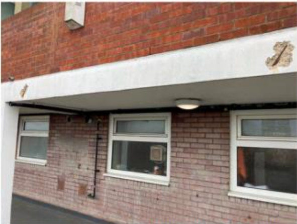
Photo 3.23: Spalling on 5 th floor slab edge visible from 4 th floor walkway between entry to 177-182 and 183-188
