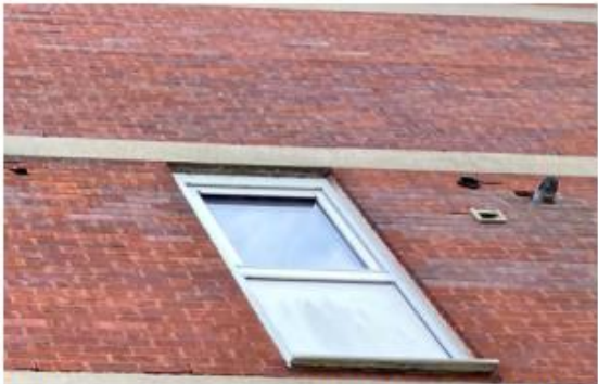
Photo 3.35: Holes in brick work on Shuttleworth Road elevation to flats 63-65
