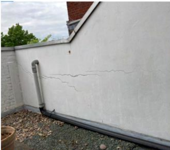
Photo 3.5: 4 th Floor Communal Terrace opposite flat 218 showing crack in side wall
