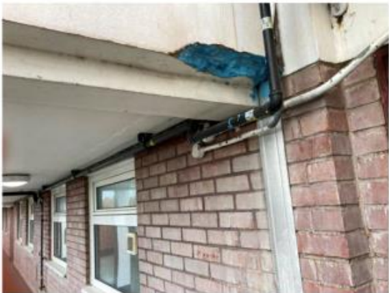
Photo 3.21: Severely spalled concrete with surface painted. Adjacent to entry to flats 177-182 at 4 th floor walkway. Same beam in photo 22.
