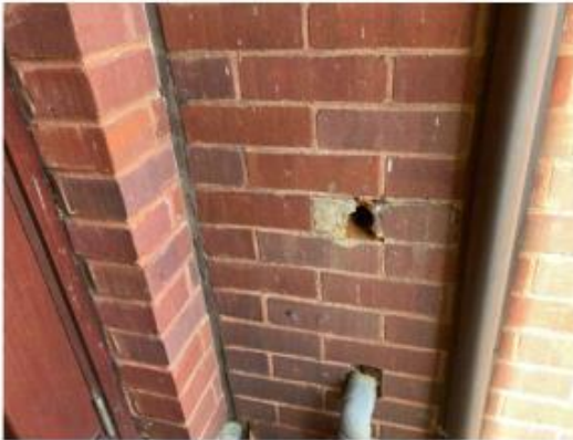
Photo 3.30: Entrance side wall to flat [redacted] facing inner green showing hole in brickwork resulting from pipe removal.
