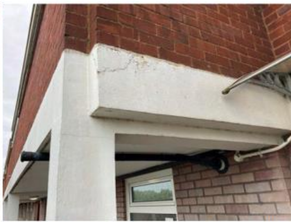
Photo 3.18: crack at top corner of beam LHS of entry to flats 165-170 at on 4 th floor walkway.
