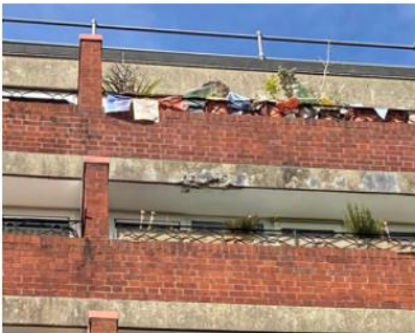
Photo 3.11: Spalling of concrete at bottom of 5 th floor balcony slab and roof beam facing inner green between sub entry to flats 37-38 and 44-43
