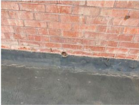
Photo 3.24: Cracked asphalt termination on wall at 4 th floor walkway.
