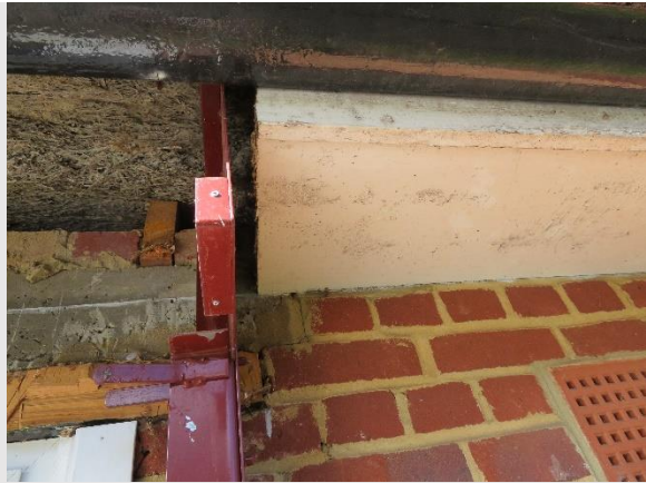
Photograph 4. Gap at soffit (area adjacent to photo 3)
