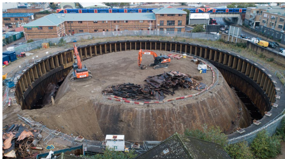
capturing the carbon from the gasholder
