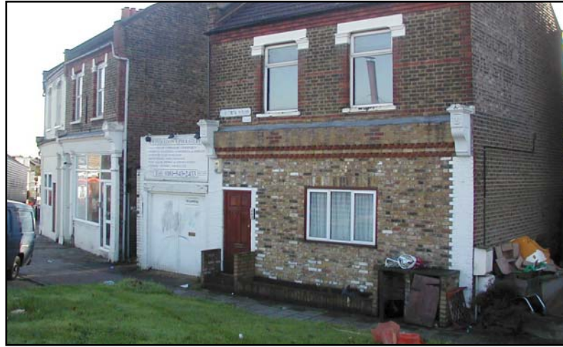
Shopfront removed: new door without fanlight inserted along with a small window with horizontal emphasis
