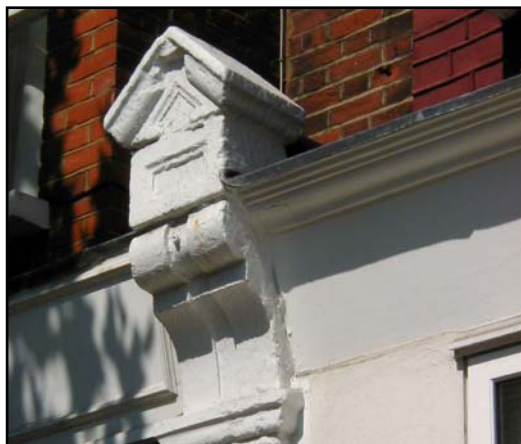
Decorative shopfront corbel retained after conversion. The shopfront fascia sign has been replaced by a band of render.
