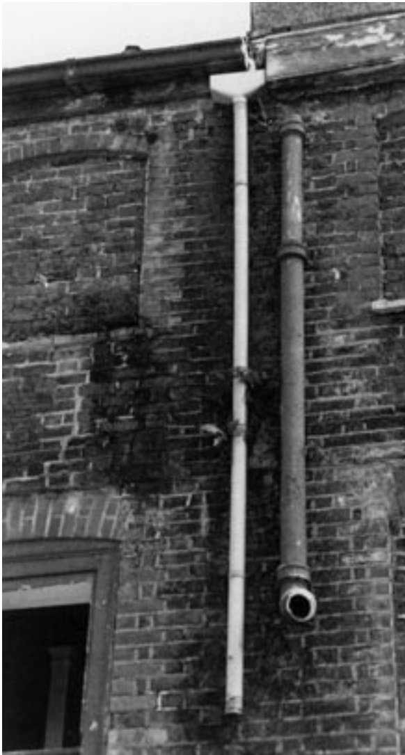
Defective gutters and pipes have caused severe damage to this listed house. (Wandsworth)
