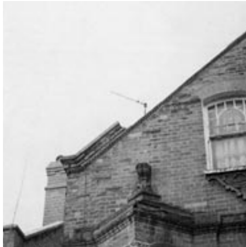
Poor brick repair and loss of the rich cornice have disfigured this house. (Tooting)
