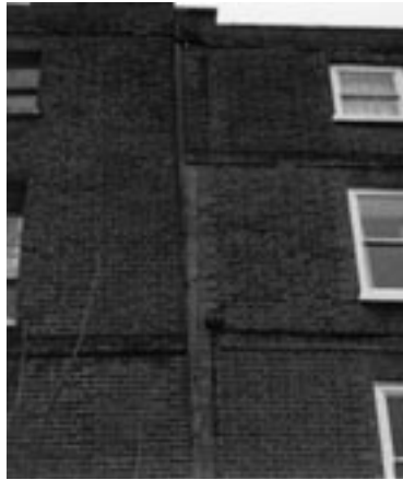
Structural cracking from long term movement can still be repaired
